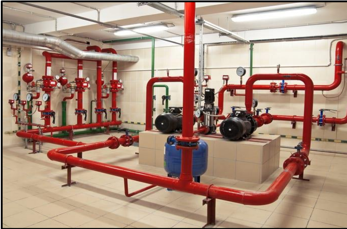
FIRE PROTECTION SYSTEM
