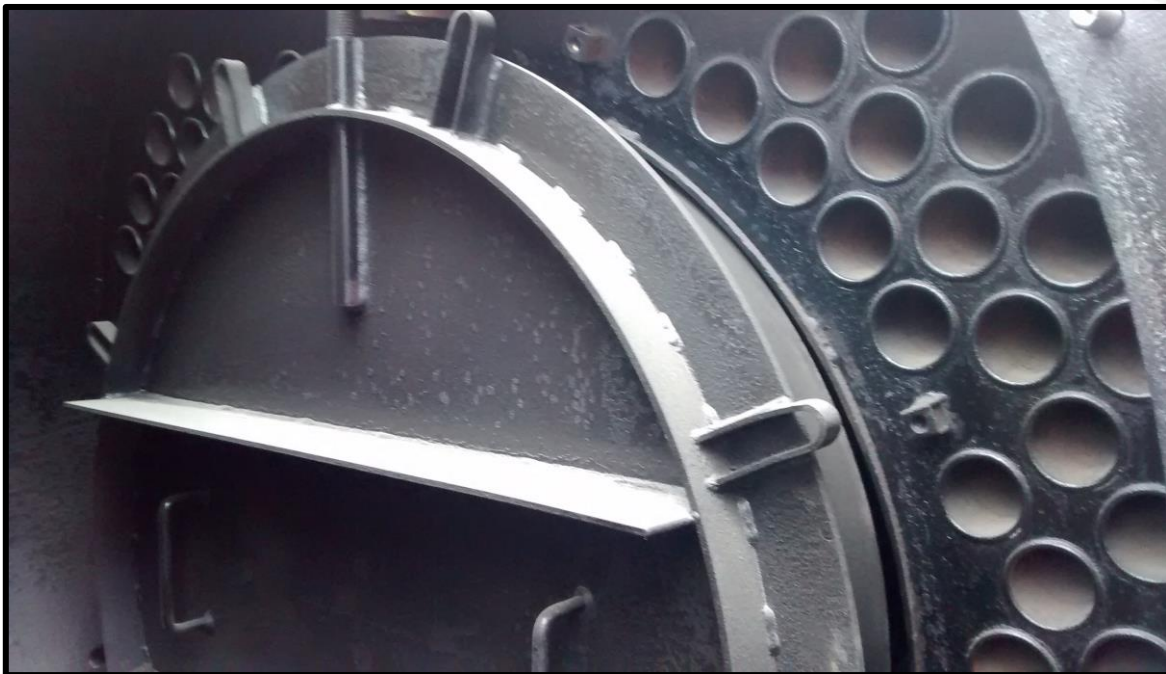
STEAM GENERATION AND HEATING PROJECTS
